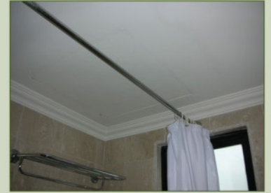
Moisture resistant ceiling and wall lining in wet area
