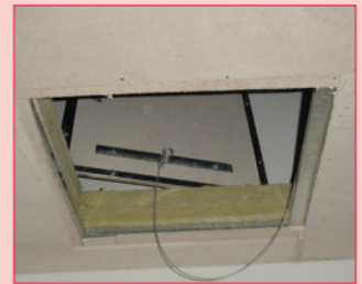
Access panels at fire rated ceiling
