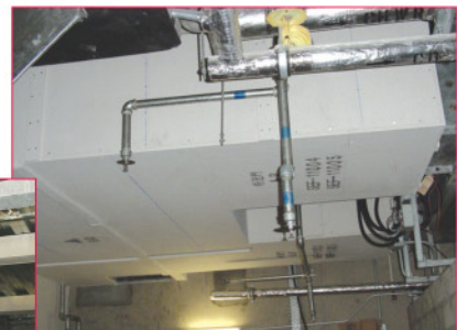
Fire rated duct
